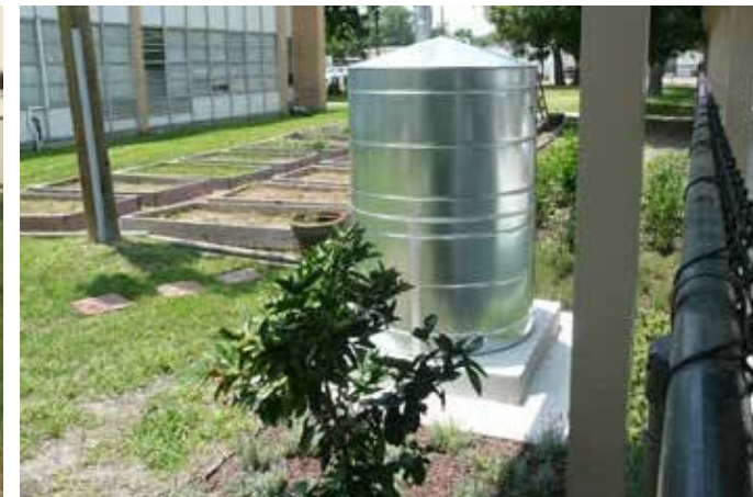
Ross Elementary rainwater harvesting
