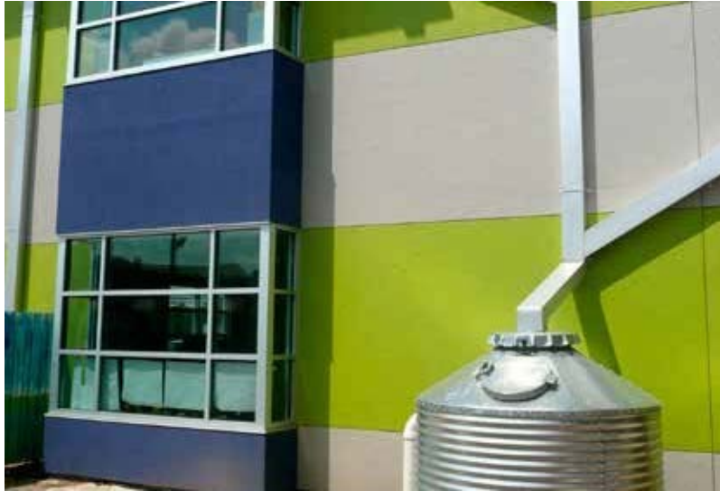
Baker Ripley rainwater harvesting
