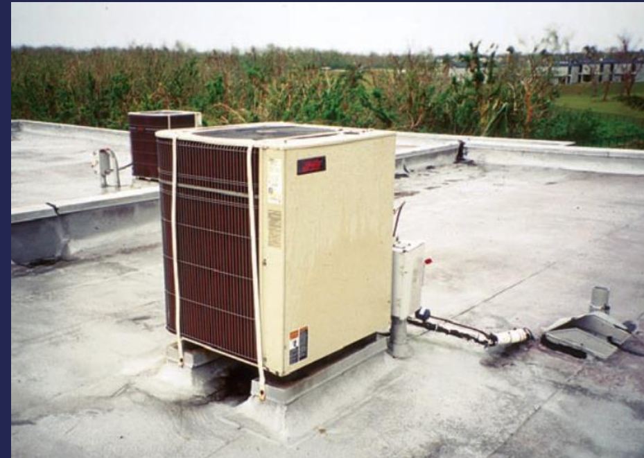
This condenser had supplemental attachment straps to hold it in place during Typhoon Paka (Guam, 1997)
