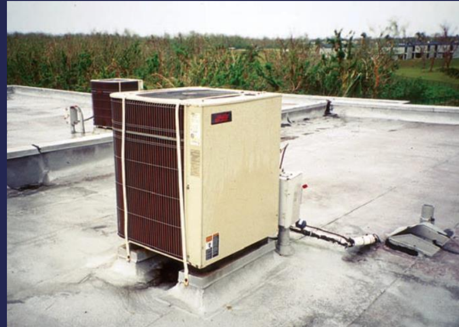
This condenser had supplemental attachment straps to hold it in place during Typhoon Paka (Guam, 1997)
