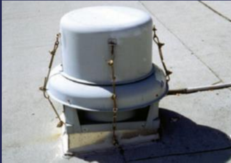
Cables were attached to prevent the cowl from blowing off. Typhoon Paka (Guam, 1997)
